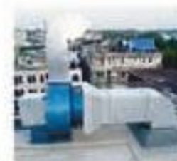
Exhaust Fresher Air Ducting
