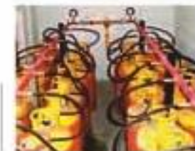
LPG Bank Pipeline/Gas Bank
